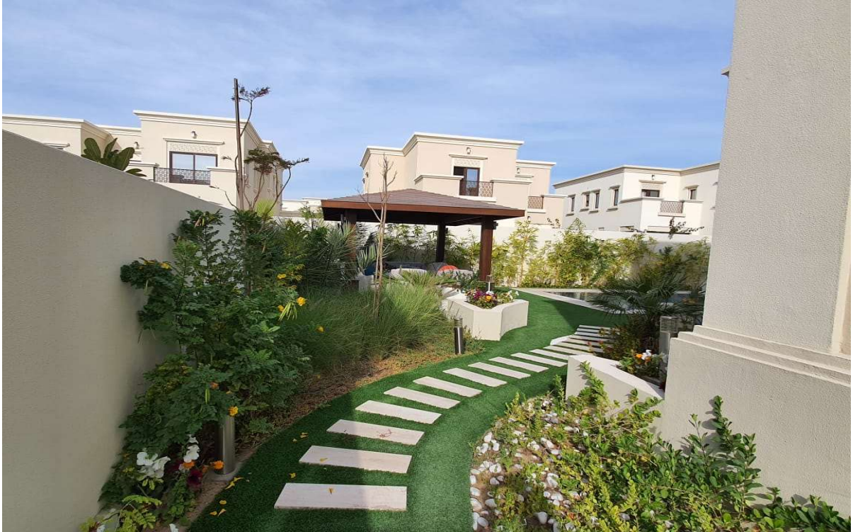
Artificial Grass with Stepping Stone work at Arabian Ranches 3rd in Private Villa
