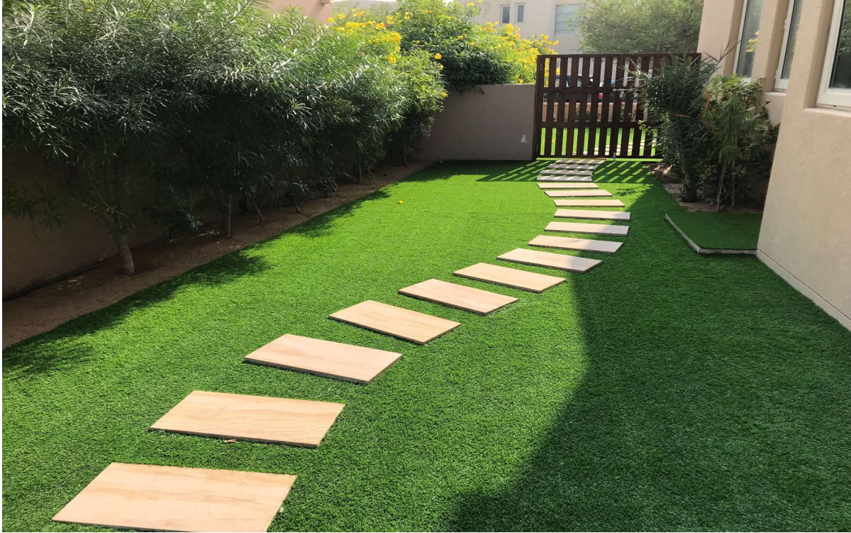
Artificial Grass with Stepping Stone work at Arabian Ranches 1st in Private Villa
