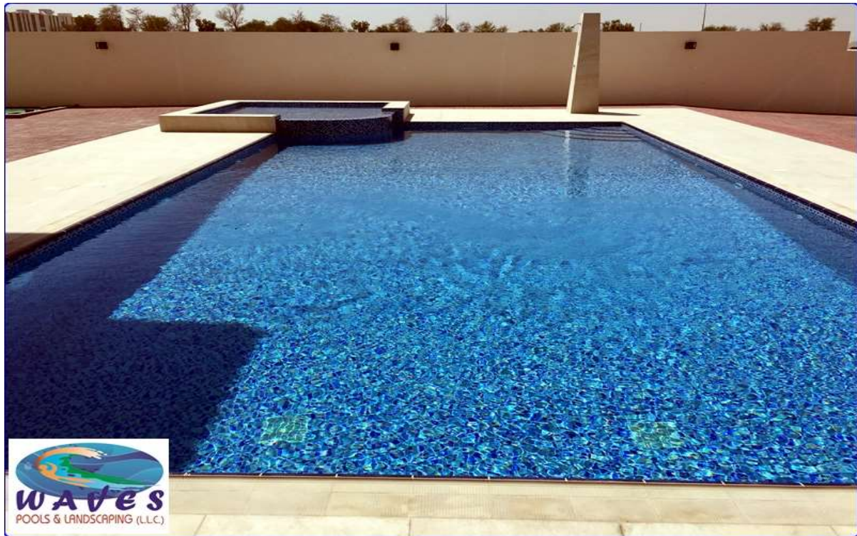
Skimmer Pool with Kid's Pool at Nad Al Sheeba in Private Villa.
