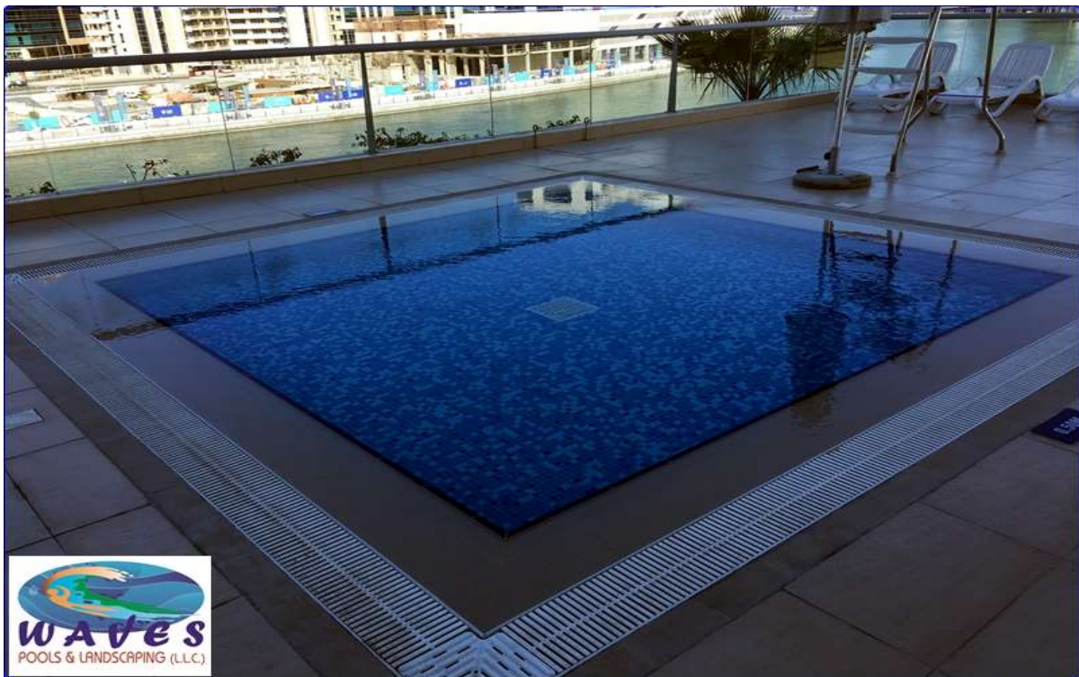
Overflow Pool with Kid's Pool at Business Bay - Client : M/s. Deyaar Developments PJSC
