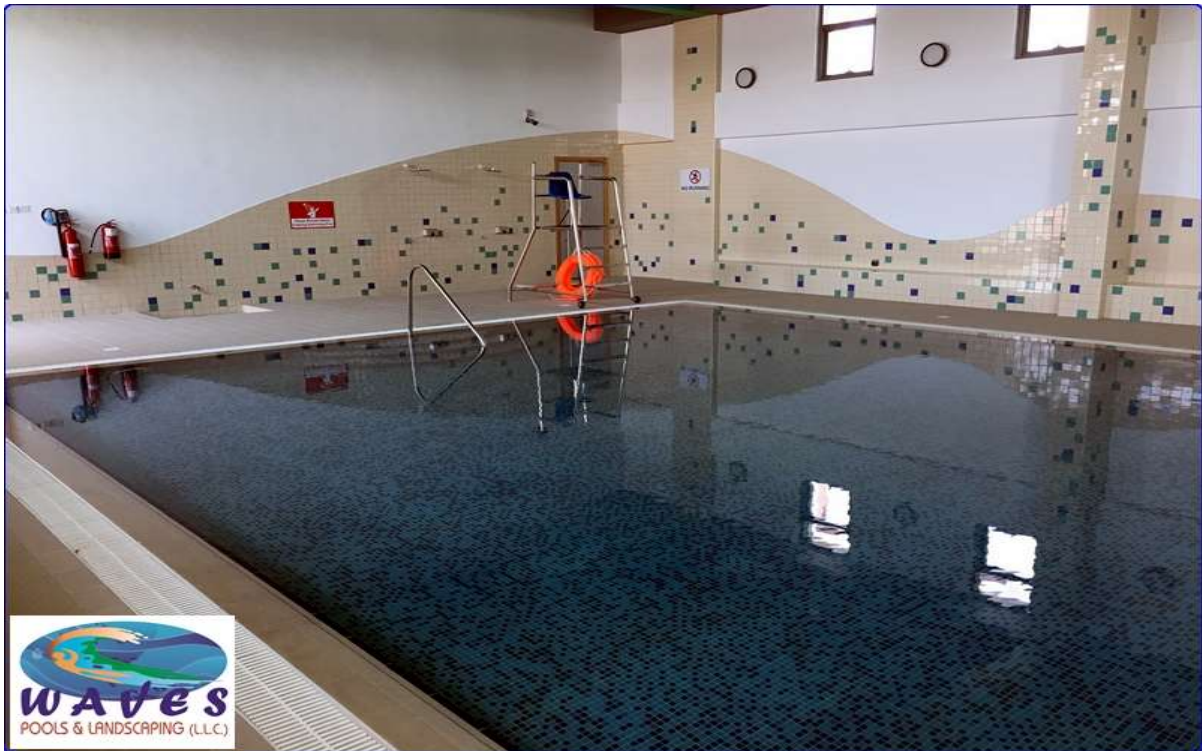
Overflow Pool at Nad Al Hamar. Client : M/s. Educational Investment International LLC, Dubai.
