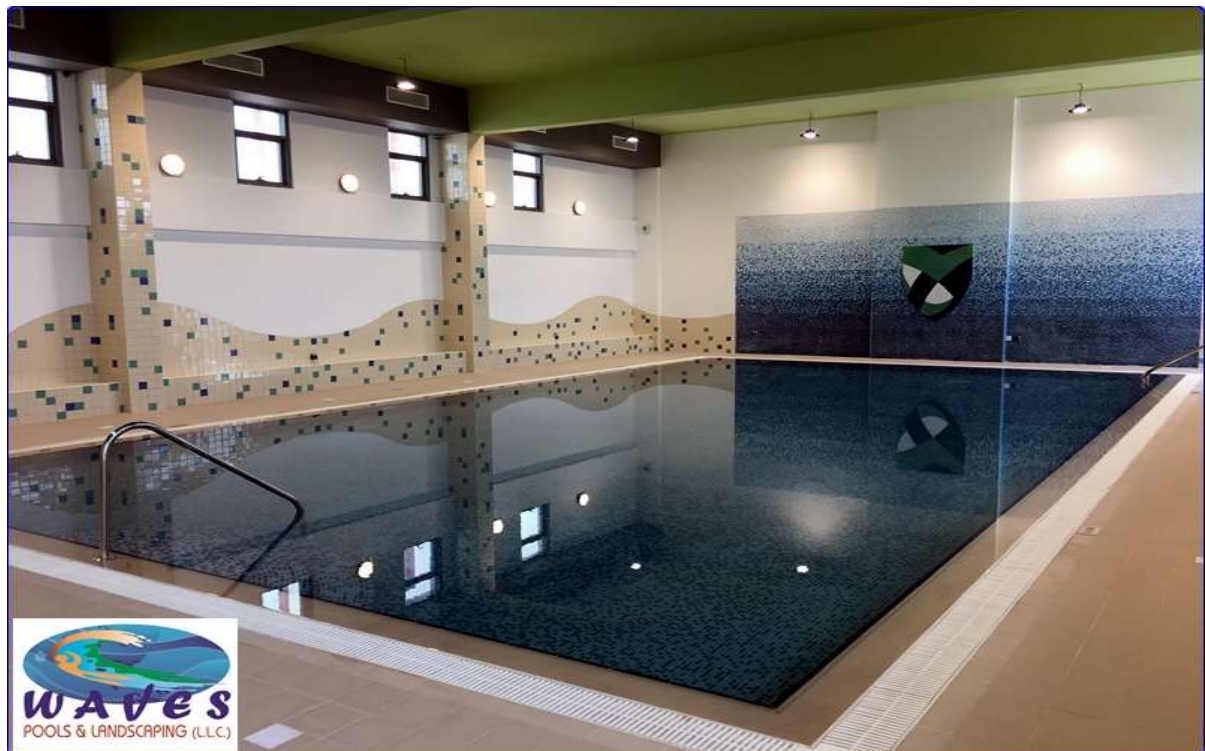
Overflow Pool at Al Barsha, Client : M/s. Educational Investment International LLC, Dubai.
