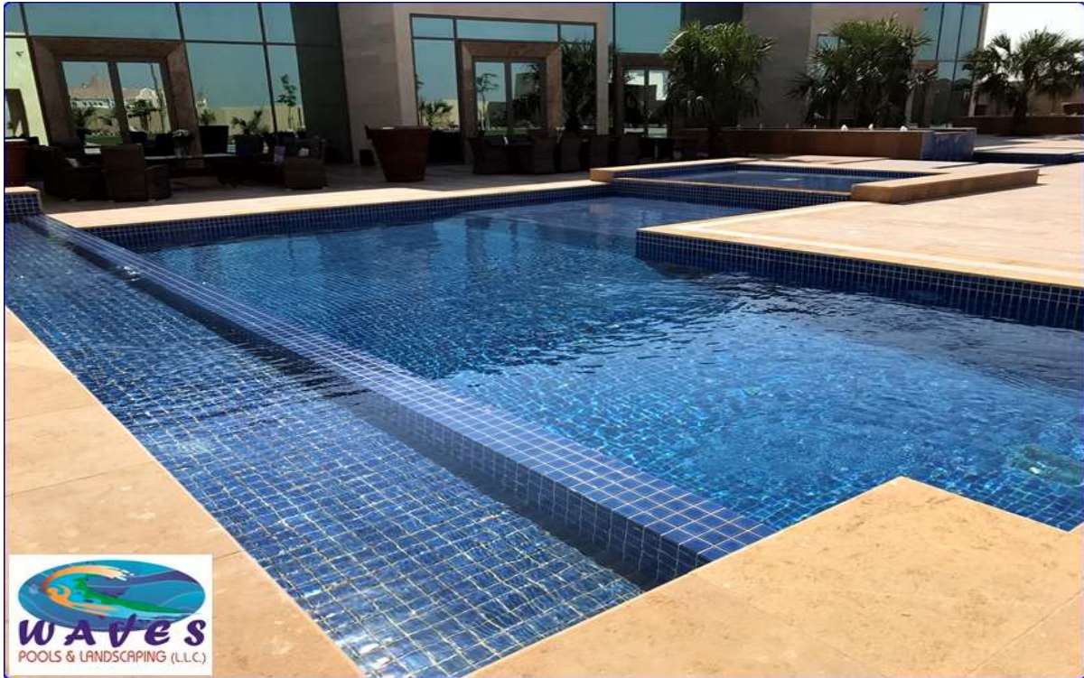
Overflow Pool with Water Body at Nad Al Sheeba in Private Villa
