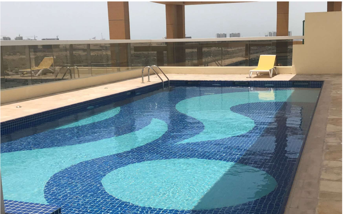
Skimmer Pool at Al Furjan in Residential Tower
