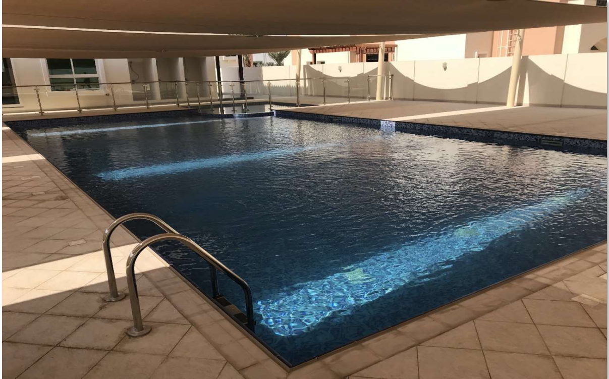
Skimmer Pool with Kid's Pool at Dubai Sports City in 35 Villa compound
